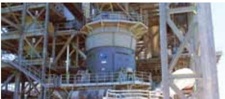
The new vertical finish mill.
