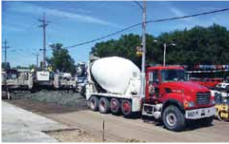
Cement from Louisville's plant is used in the re-pavement of a Louisville street.
